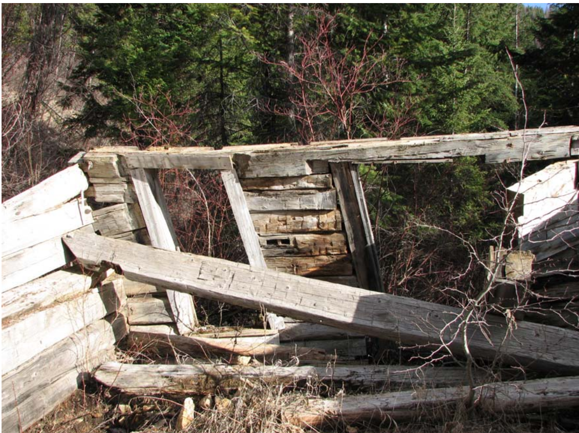
Figure 7. Cinkers/Louiseville Structure 3. Photo taken during Spring 2007, note decay since 1995. Photo by Author.
