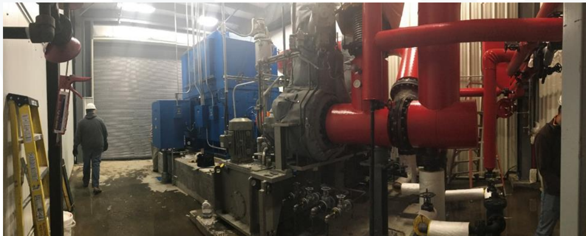
A very similar 3 MW steam turbine generator installed in a small steel structure.
