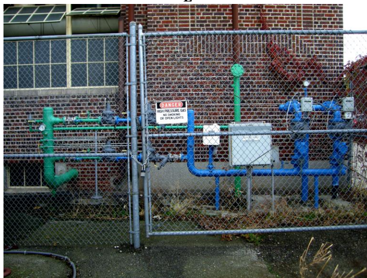
Natural Gas Service Entrance - North Side of Boiler Plant
